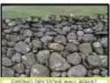
EXISTING DRY STONE WALL BUILT BY HOUSING DEVELOPER AS PART OF COMPLETED HOUSING DEVELOPMENT
